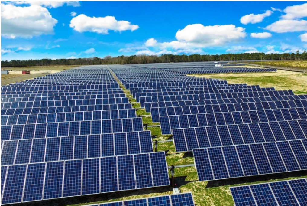
Figure 29 - Many arrays in a PV solar power plant ( MIT News, 2020 ).
