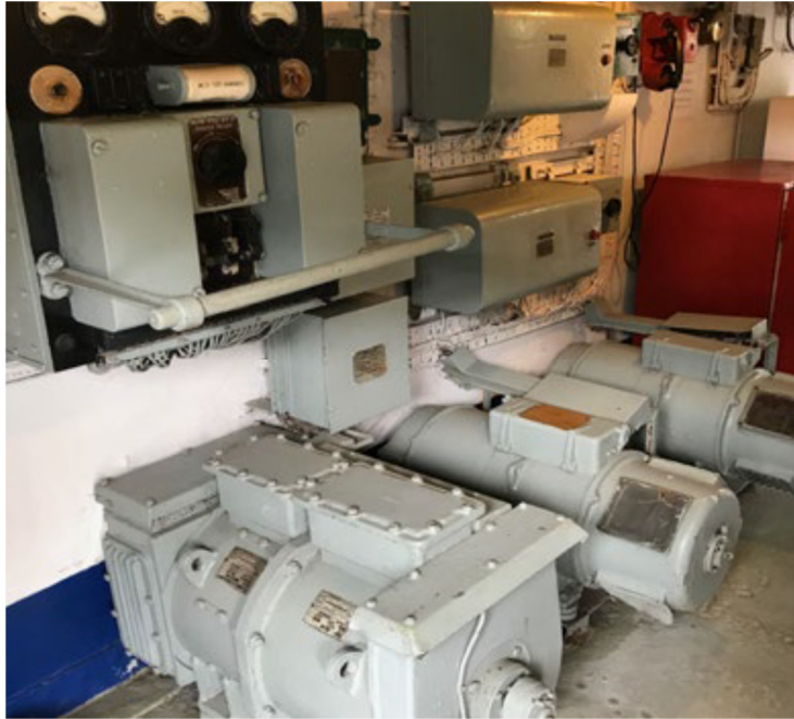
Figure 10 - Ship rotary inverter.
